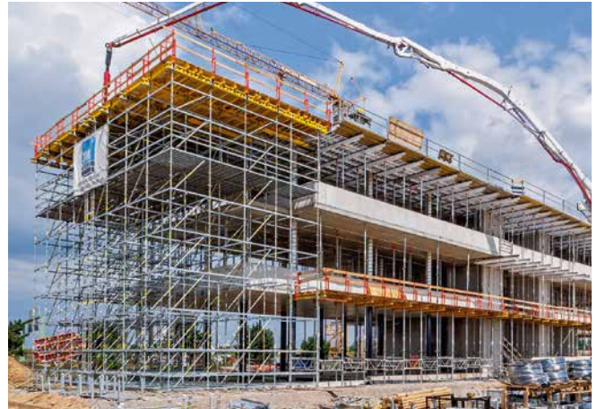
Complete solution from one source: wall and slab formwork as well as the shoring and reinforcement scaffolding were optimally adapted to match the project requirements.
