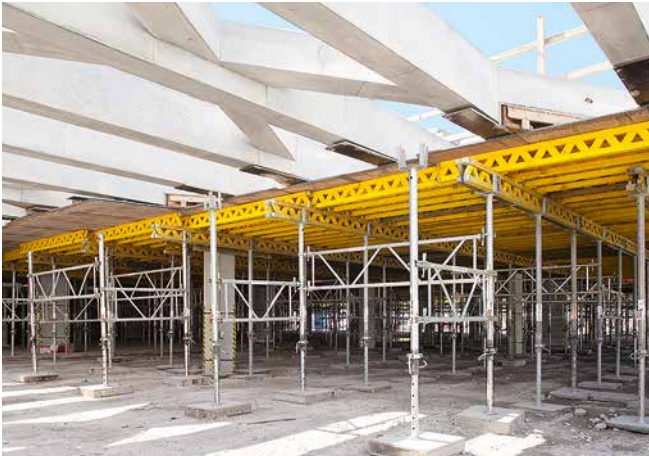
MULTIFLEX served for the construction of the cast-in-place beams with the PERI Props connected by means of PRK Frames to form shoring towers.
