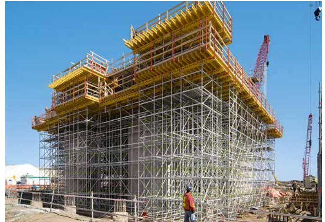
With PERI UP Rosett and MULTIFLEX, the high loads from the massive structural elements at heights of between 10 m and 12 m were reliably transferred into the ground.
