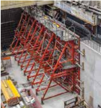
The required working platforms are correspondingly attached to the respective formwork system.
